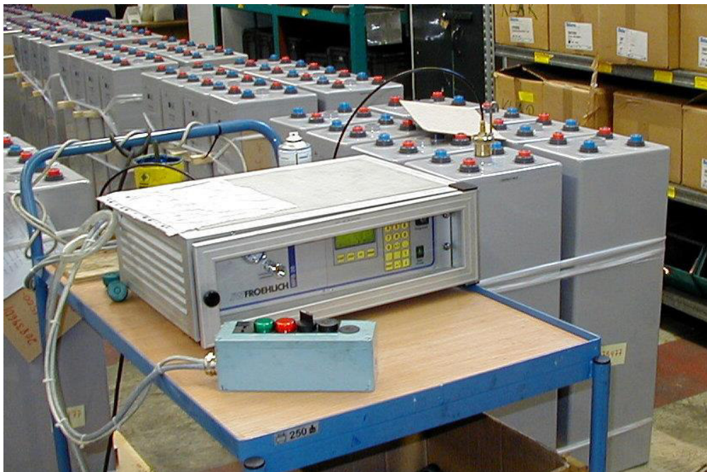
Figure 30 – Tightness test of 12 OPzV 1500 single cells.
