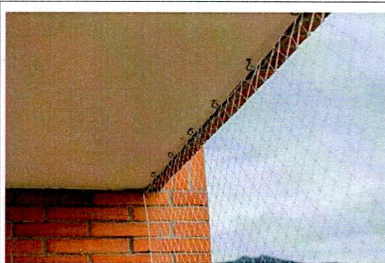
MALLA NYLON INSTALADA
