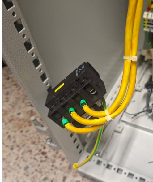
Figura 5b: Interruptor general
