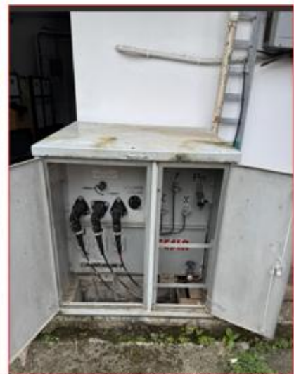
Transformador Pad Mounted de 30 KVA-220 V./2.4 KV.
