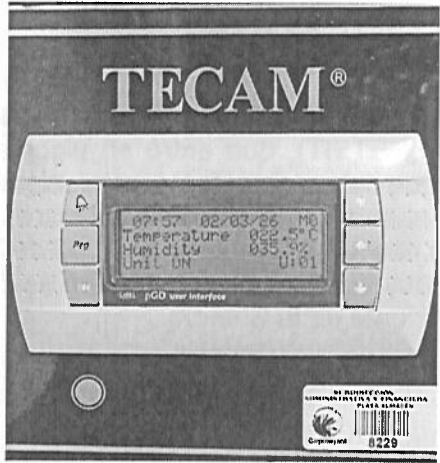
Panel de control
