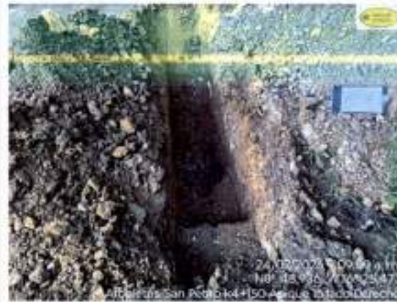
Apique No. 16 K4+150
