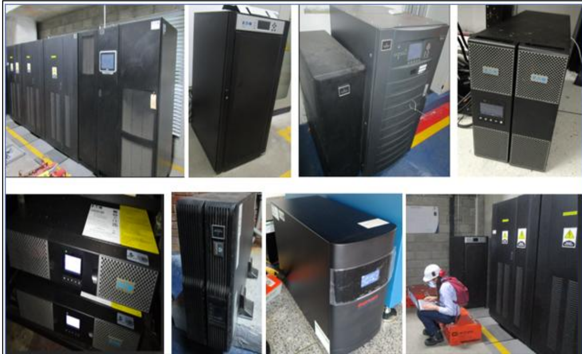
Sistemas de UPS ((Uninterruptible Power Supply)).
