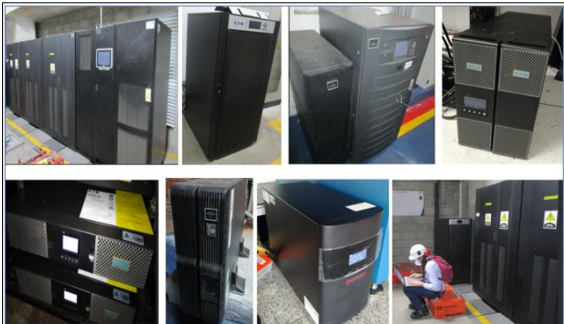
Sistemas de UPS ((Uninterruptible Power Supply)).
